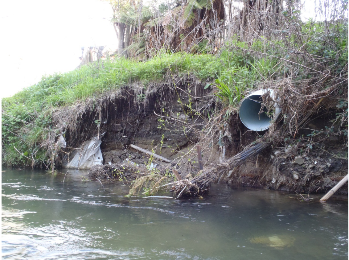
Figure 6. A recently installed drain (Site 1 true right bank) without adequate bank reinforcement.
